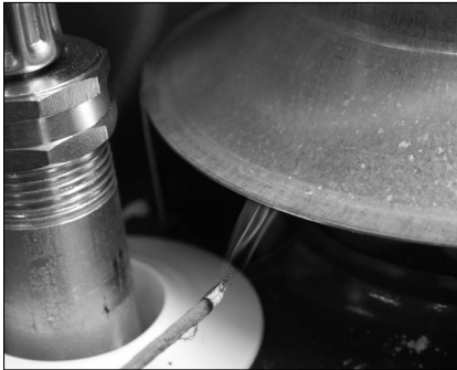
Figure 35 - Test the air supply and vent to make sure the water heater has adequate air and is venting properly.
